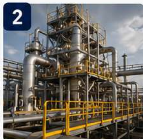
2 ACID GAS TREATMENT
